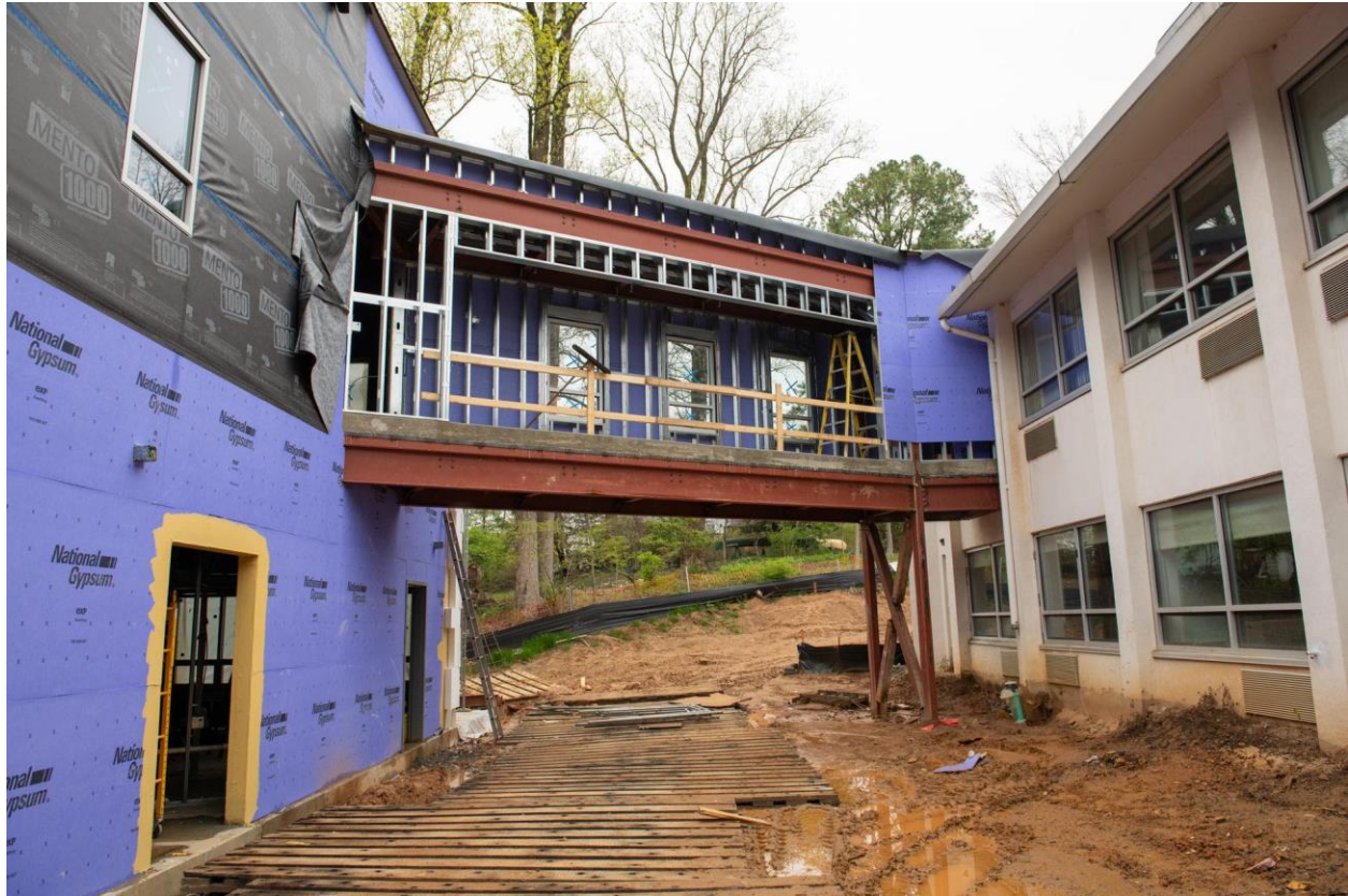
As for the Small Sanctuary addition, work has begun on the roof. The picture below was taken from the foyer right outside of the Small Sanctuary, looking up. You can see the wood beams and the ceiling and the framing for the skylights that will be installed. It will be a gorgeous space!
